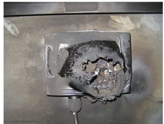
Junction box failure in the field. Photo courtesy of Photovoltaik Buero.
